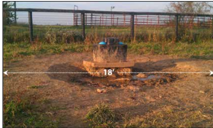
Figure 3-2. Without an all-weather surface, the heavy use area has eroded to the point where the watering facility is almost inaccessible and is no longer frost-proof. The depression also poses a threat to livestock health because livestock have to stand in mud and excrement to drink. Note the diameter of the bare soil area (18'). Photo by Jeff Lehmkuhler
